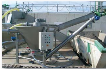
Grit Washing Plant
