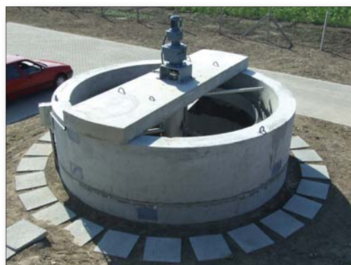
Gravity Sludge Thickener
