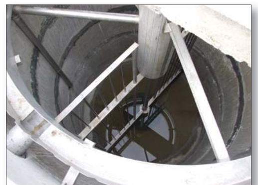
Gravity Sludge Thickener
