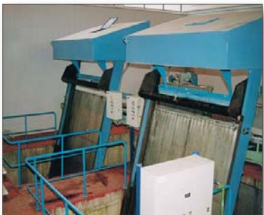
Automatic Cable Screen
